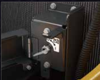
Battery Disconnect Switch with DEF Purge Notification Buzzer
